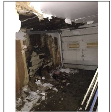
Above: The interior of the garage showing severe deterioration and mold issues. 09/12/2019
